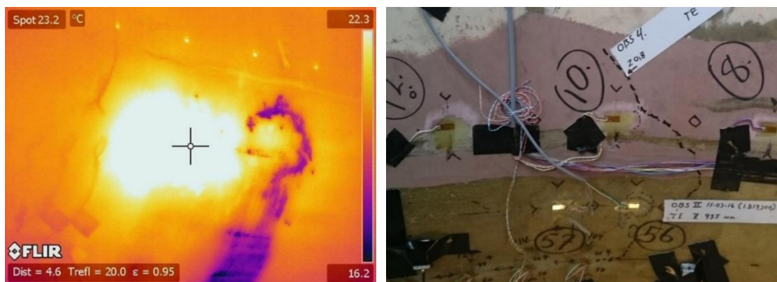
Figure 17: NDT (Ultrasound) inspection was used to detect the size of the damage in the Root-Transition zone of the SSP34m blade.
