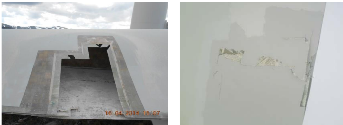
Figure 55: Extract of a blade inspection report showing transverse cracks in the max chord region on an infield wind turbine blade.
